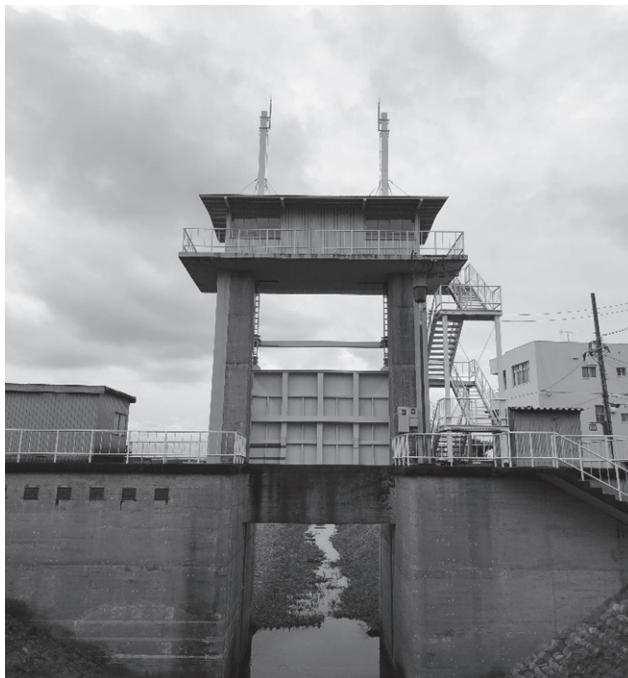
Figure 6. Flood Control Gates in Gifu City, Gifu Prefecture Author' s Fieldwork in Gifu Prefecture, Japan, 2019
